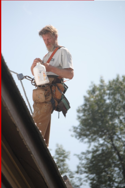
Roof repairs were part of the facelift given to St. Felix Mission in Stewart this past summer.
